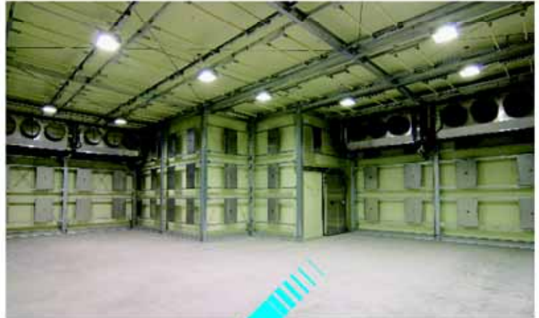
Large size freezing warehouse freezer with harmonic oscillating function (2000m x 6m)
